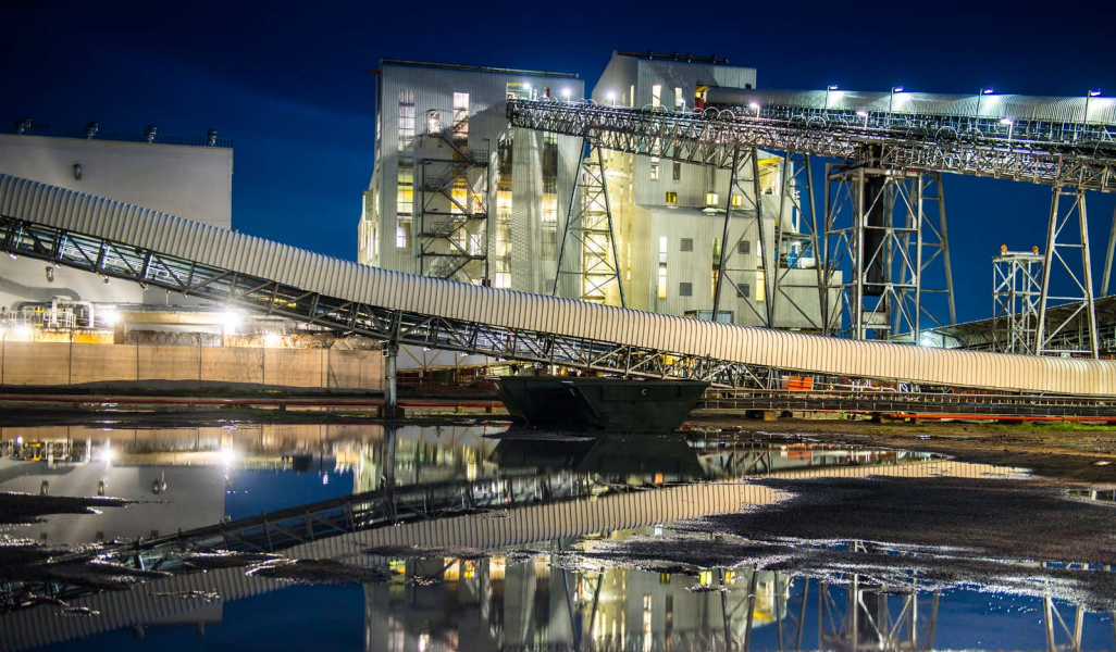
XRT (X-ray transmission) circuit buildings and processing plant
