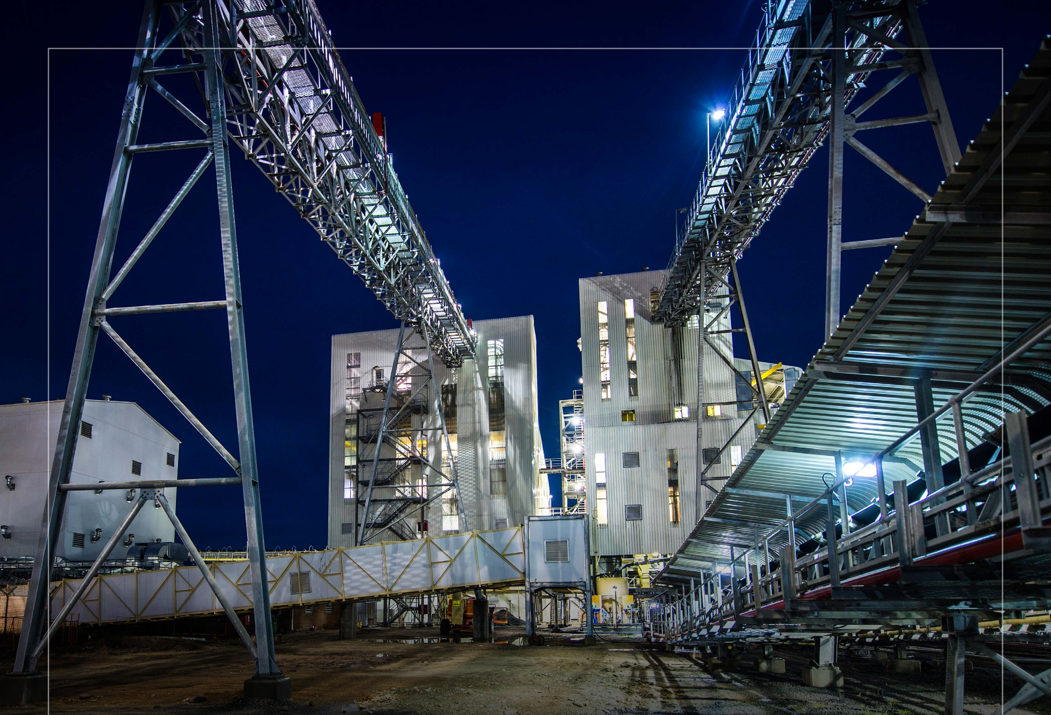
Conveyors leading to main XRT (X-ray transmission) buildings
