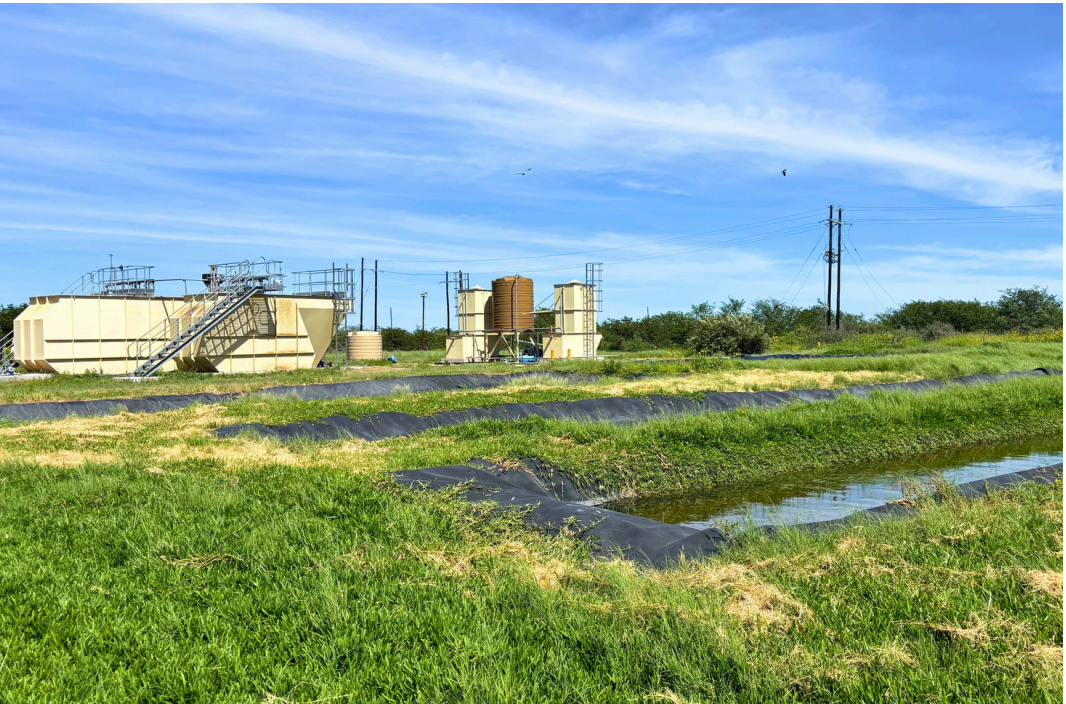
Wetlands wastewater treatment
