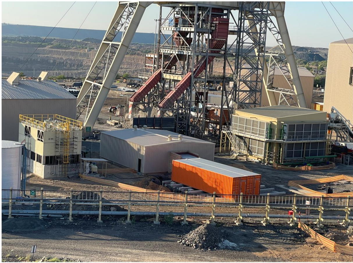
Bulk Air Cooling System
